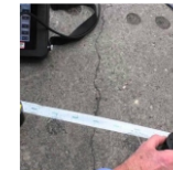
Crack Depth & Crack Bar Monitoring
